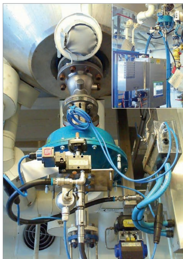
Above: SchuF valve with integrated Mettler Toledo ReactIR™ FT-IR probe installed at the outlet of a reactor. The probe is connected to an online reaction-monitoring instrument.
